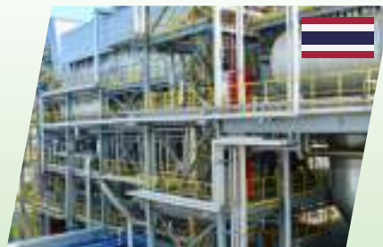
Waste-to-Energy Power Plant
