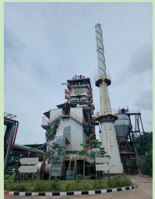
Biomass Boiler, Cement Industry
