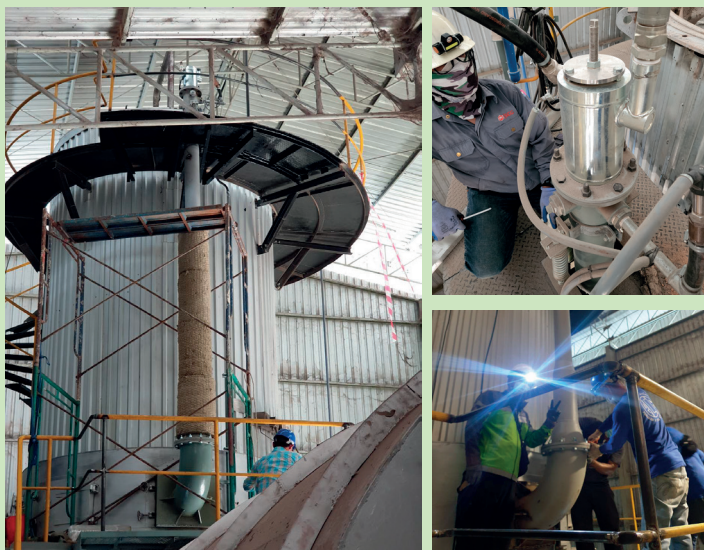
Online Cleaning Biomass Boiler (Infrasound), Rubber Industry
