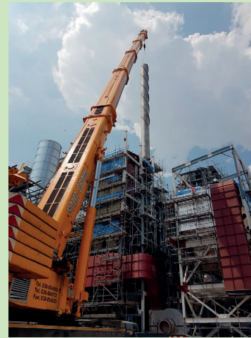
New Green Boiler, Food Industry
