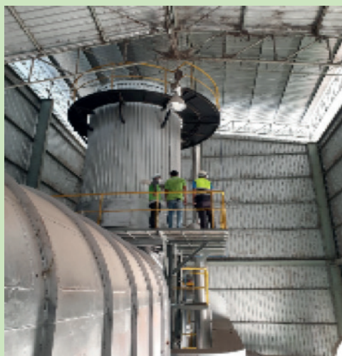
Biomass Boiler Infrasond, Rubber Industry
