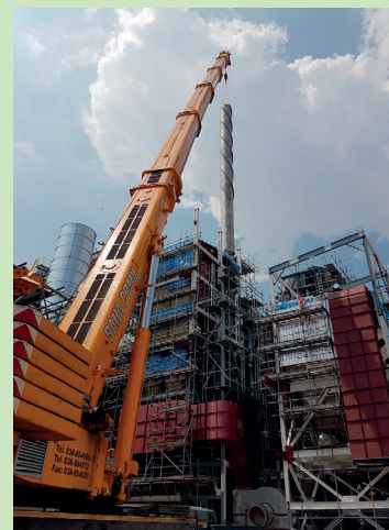
New Green Boiler, Food Industry
