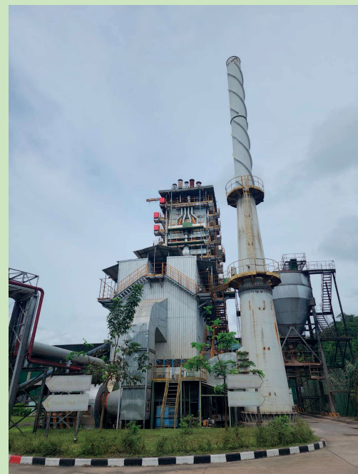
Biomass Boiler, Cement Industry
